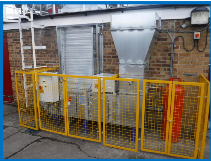
TYPICAL HEATER INSTALLATION C/W SECURITY CAGE / LPG STORE
