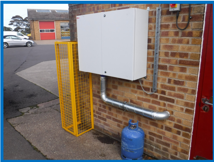
SMOKE SYSTEM SUPPLYING 1FLOOR c/w CYLINDER CAGE
