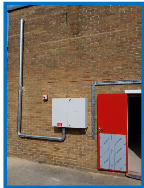
SMOKE SYSTEM SUPPLYING 2 FLOORS
